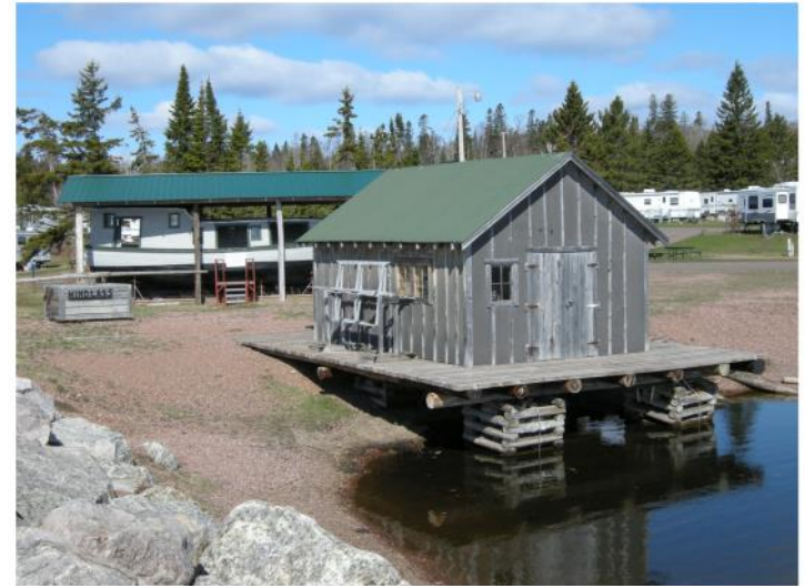
Near-term protection and preservation of the Neegee is a priority. Fish house replica cribbing must be inspected.
